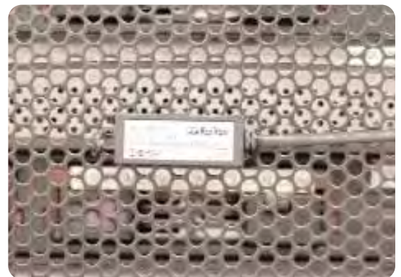
An example of a temperature sensor mounted at the cold air inlet of a server rack. Sensor is connected to an intelligent PDU (not shown).
