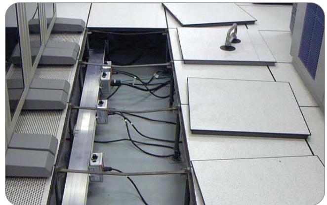
A clean, organized power busway system simplifies power distribution and can lower HVAC costs.
